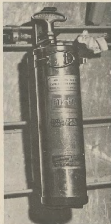
Carbon Tetrachloride (Pyrene) type extinguisher located beside rear entrance door.
