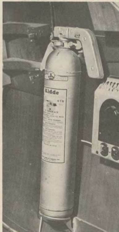
CO 2 type extinguisher located in aft pressurized compartment, aft of auxiliary equipment panel.
